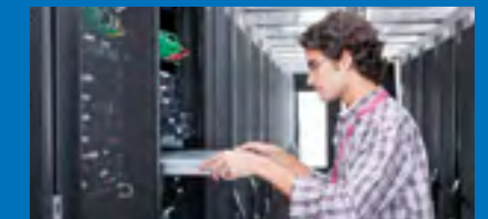
Backup Power UPS
