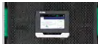
Green light bar showing healthy UPS
